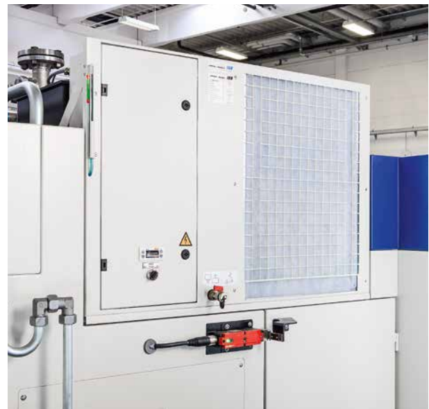
Machine cooling unit
